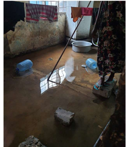
Figure 3.4 Storm water inside the house – Makuburi Kibangu
